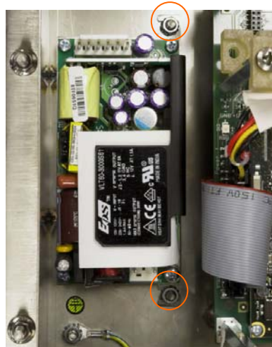
Figure 3-64: Power Supply, Disconnected
