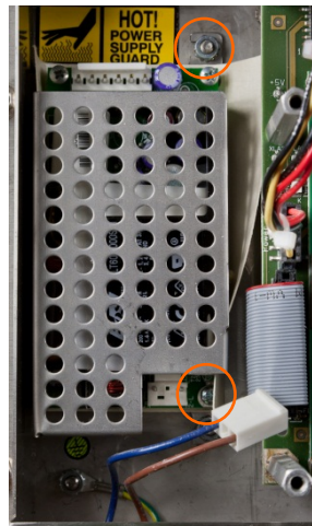
Figure 4-63: Power Supply, Disconnected
