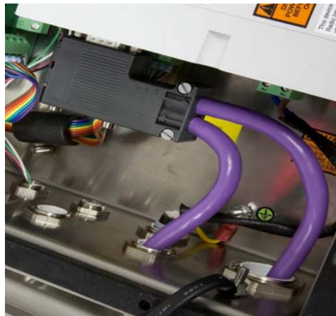
Figure 2-62: Original J-Box Enclosure PROFIBUS Cable Routing
