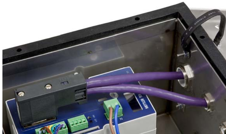
Figure 2-63: Updated J-Box Enclosure PROFIBUS Cable Routing
