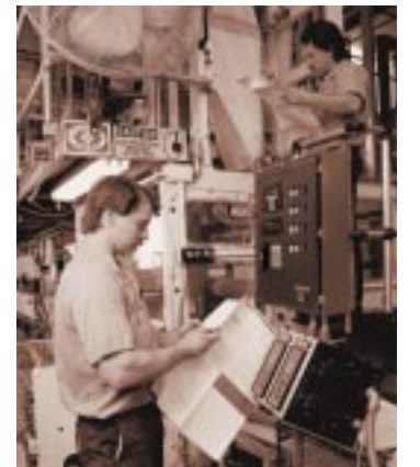
Technicians make final schematic checks on a custom ink control system during installation at a leading U.S. newspaper.
